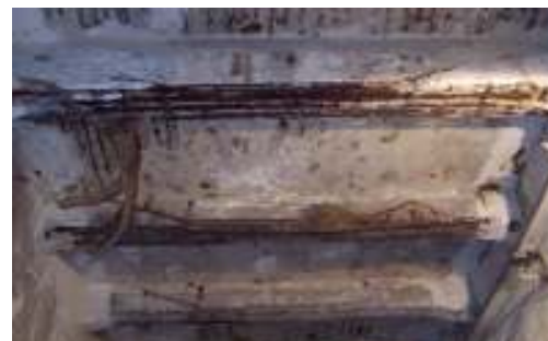
Degradation of the slab and beams of the first floor at the access tunnels
