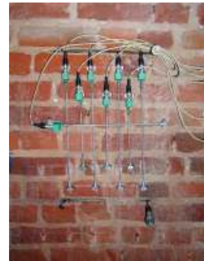
Double flat-jack test (stress-strain behaviour) on West side of the Monza Tower (Binda, 1998)
