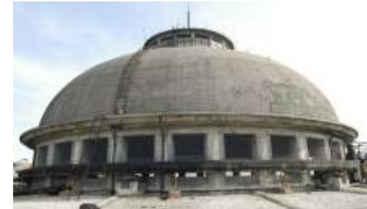
General deterioration of the rc dome.
