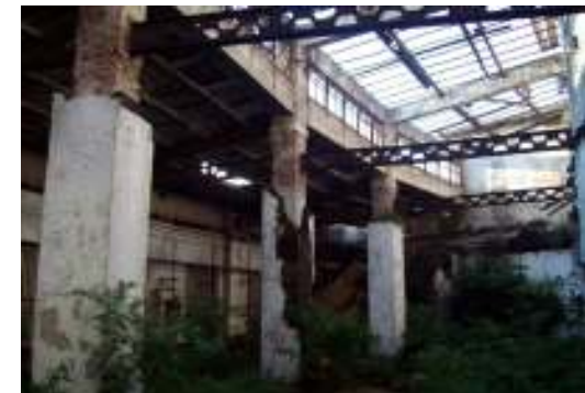
Steel roof degradation on the external ring
