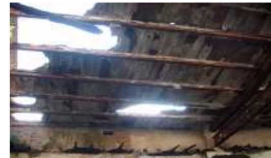
Roof degradation on the external ring
